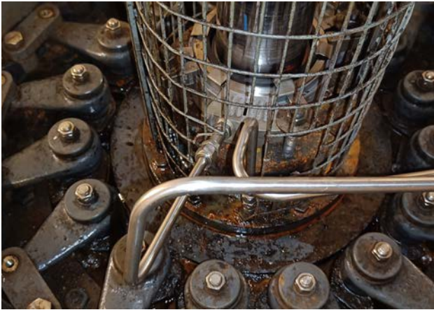
Guide Vane Mechanisms before refurbishment
