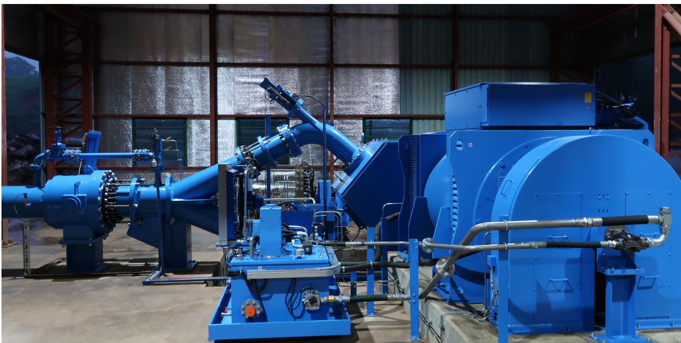
Ndiza turbine & generator
